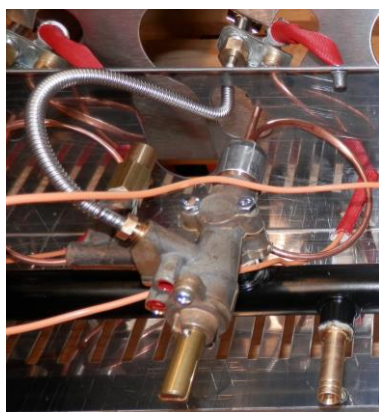
GAS CONTROL VALVE ASSEMBLY. PHOTOGRAPH 35.
